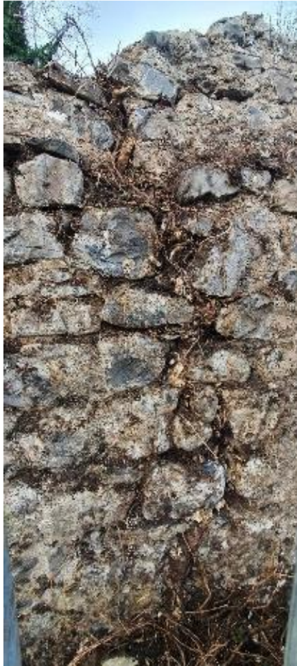
Figure 11 – Vertical crack in southeast flank wall due to roots
