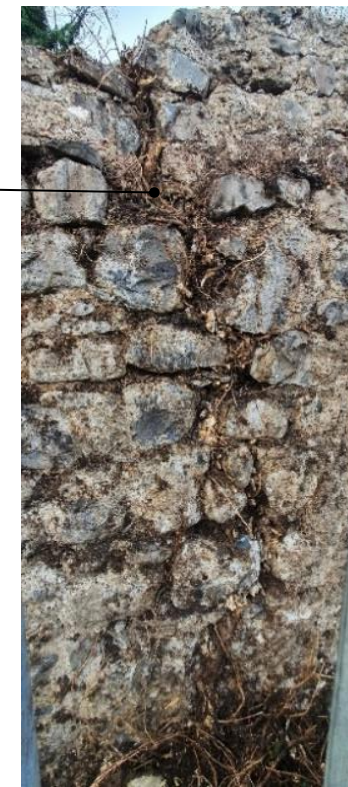
Outer face of South-East Flanking Wall showing vertical cracks
