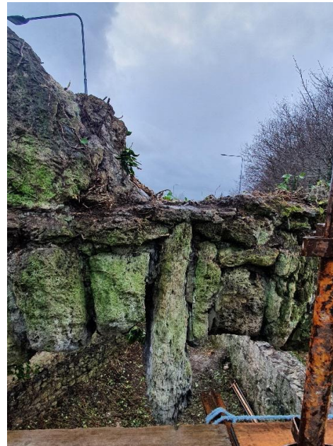
Figure 4 – Stone missing above arch keystone can be seen in the northeast elevation of the arch
